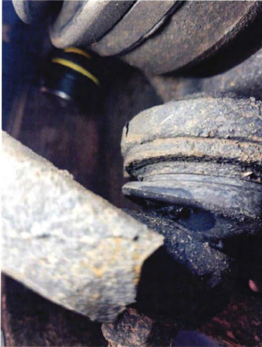
Ball Joint Condition
