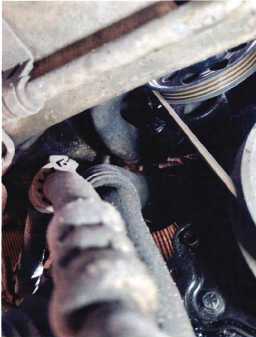
Drive Belt Condition
